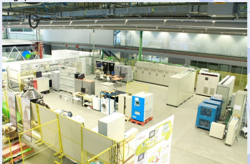
A view of an ISGAN member test facility: The Microgrid test laboratory at Technalia, Spain.
